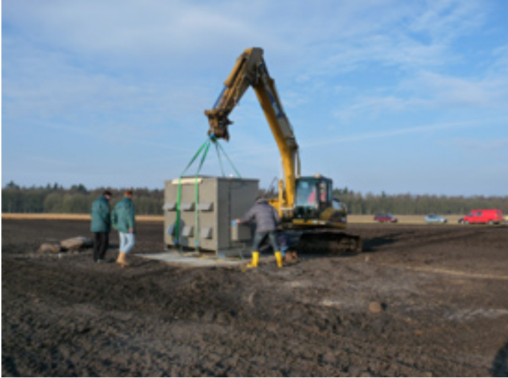
The placement of a cabinet filled with electronics at the edge of the first LOFAR station CS302. Credit: Henri Meulman, ASTRON
