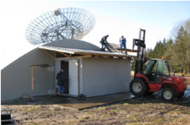
Installation of the back-end cabinets at the WSRT.
