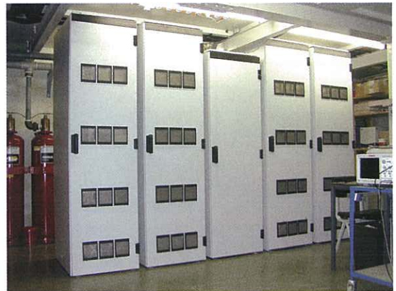
Figure 2.28 The four IVC-Cabinets and central Control and LO-distribution Cabinet, installed in the basement of the WSRT main building.
